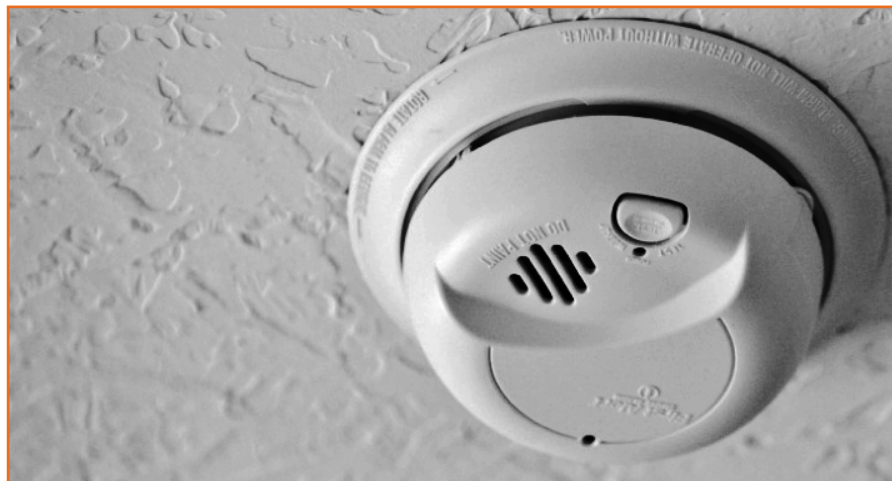
Figure 3.1 Smoke alarm on ceiling Source: Nationwide Children's Hospital, Columbus, USA
