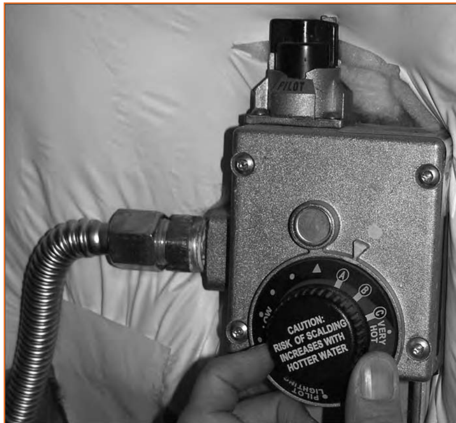
Figure 3.2 Setting the temperature on a hot water heater Source: Michael Peck
